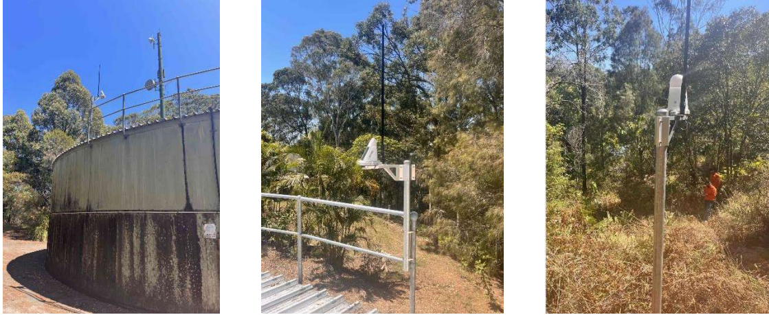
Figure 6 Site 1 photos. Left panel: base station on the top of water tank; Center panel: base station; Right panel: monitoring node.
